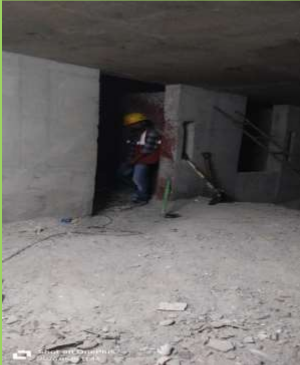
Tower-A, Lift Lobby-02, B-2 Level, Lift pit No 02 debris removal and cleaning works are in progress
