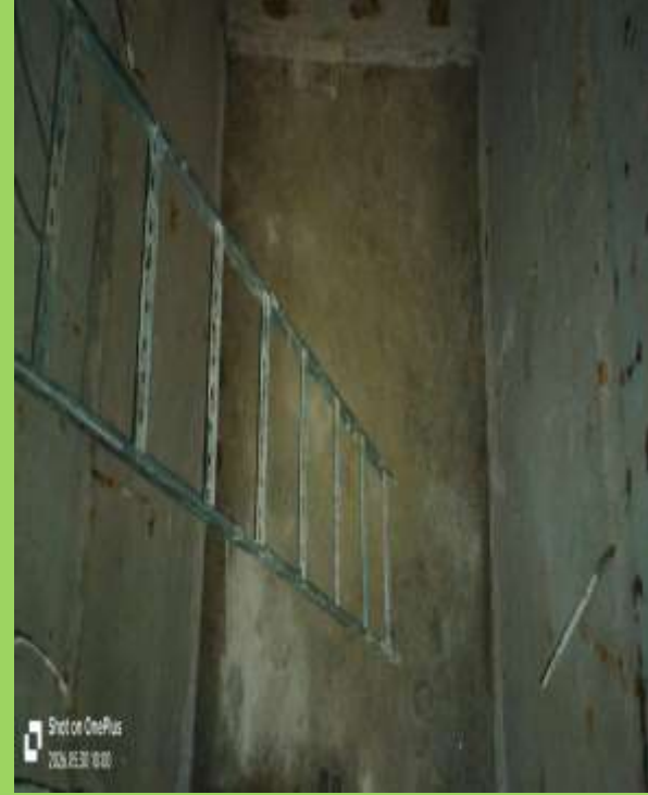
Tower-A, Lift Lobby-02, B-2 Level, Lift pit No - 02 debris removal and cleaning work completed
