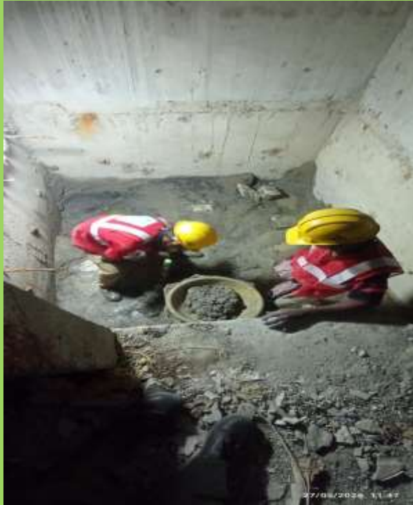
Tower-A, Lift Lobby-02, B-2 Level, Lift pit No- 02 debris removal and cleaning works are in progress
