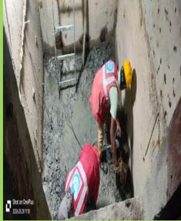
Tower-A, Lift Lobby-02, B-2 Level, Lift pit No - 02 debris removal and cleaning works are in progress
