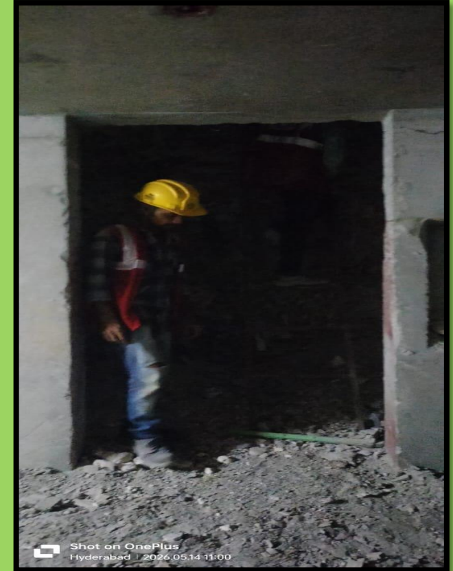
Lift Lobby-02, B-2 Level, Lift pit No 02 debris removal and cleaning works are WIP
